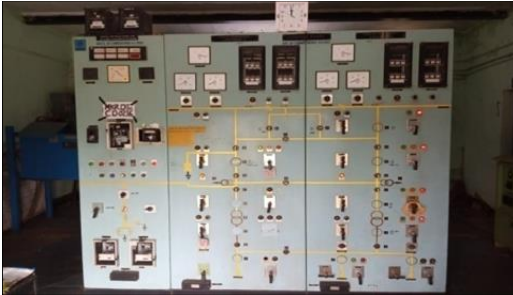
Figure 4 Control and Relay panel with Electromagnetic Relays
